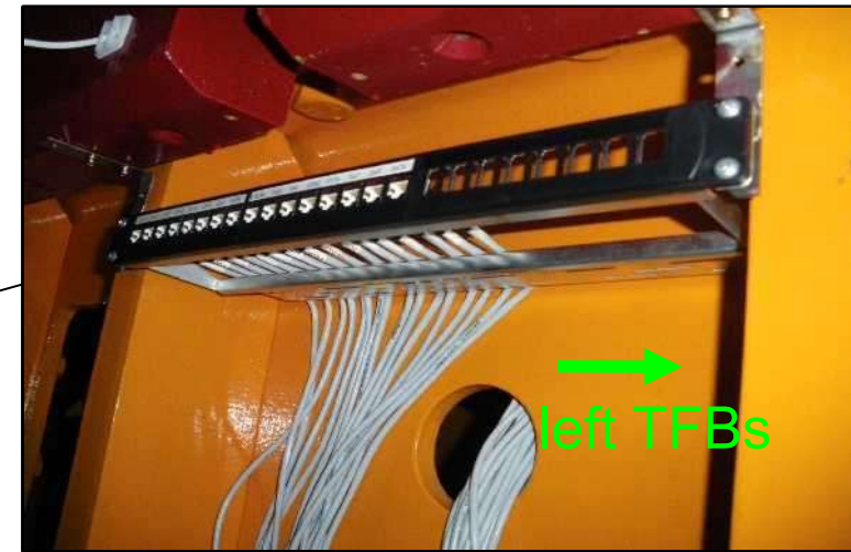
Patch Panel on left magnet support structure
