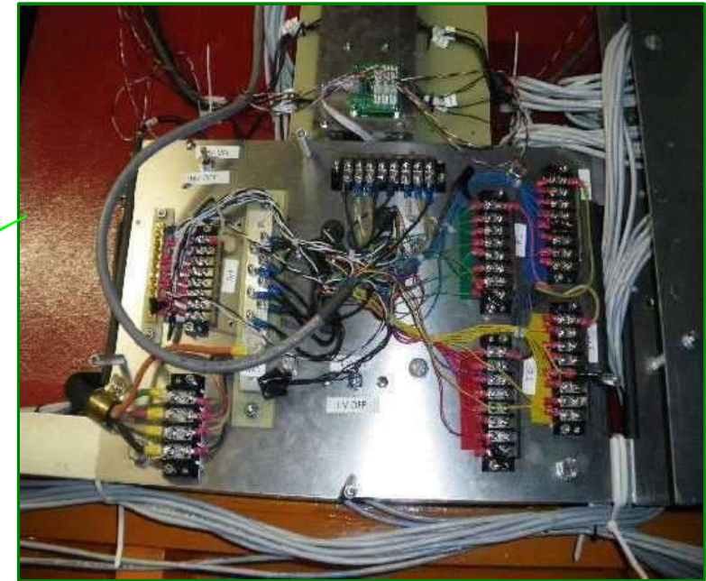
Secondary Power Dist. Boards
